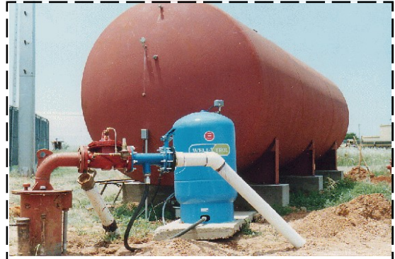
86 gallon tank replaces 10,000 gallon tank
